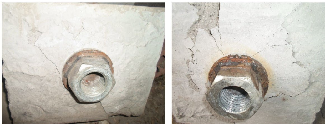
Figure 7. Failure of specimens IPE6C, IPE8C.
